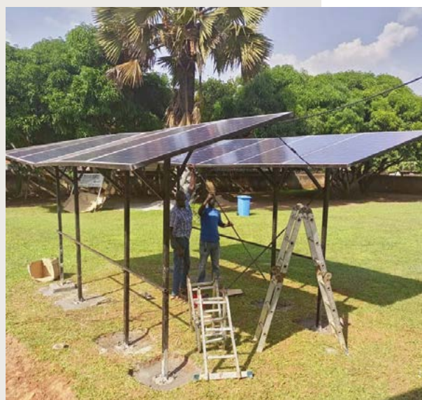
Installation of solar panels at OHCHR in Panama and in Uganda. © OHCHR
