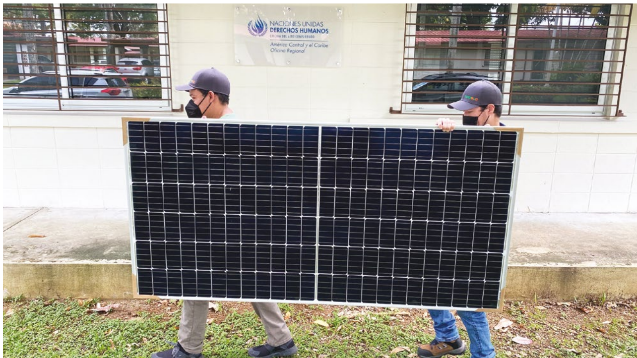
Installation of solar panels at OHCHR’s Regional Office for Central America in Panama. © OHCHR
